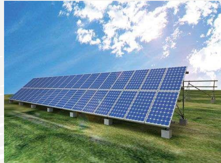
Small PV power plant
