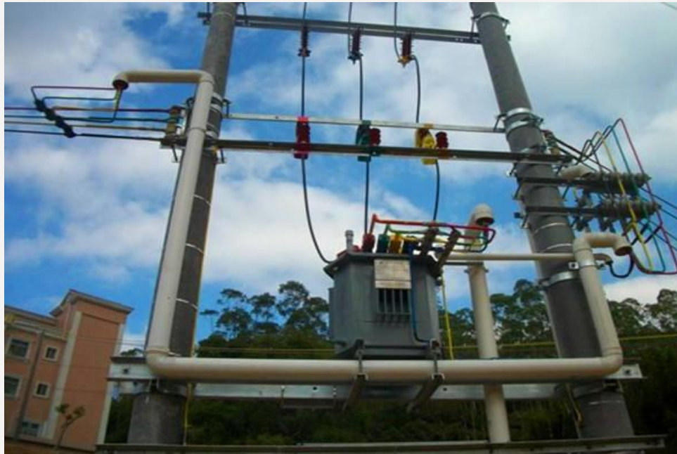
Distribution grid facilities
